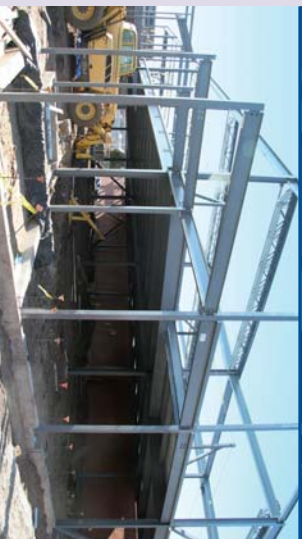
A 20,000-square-foot expansion begins to take shape at the New Britain site of the Community Health Center. The two-story expansion will add 16 additional medical exam rooms to the facility on Washington Street.
